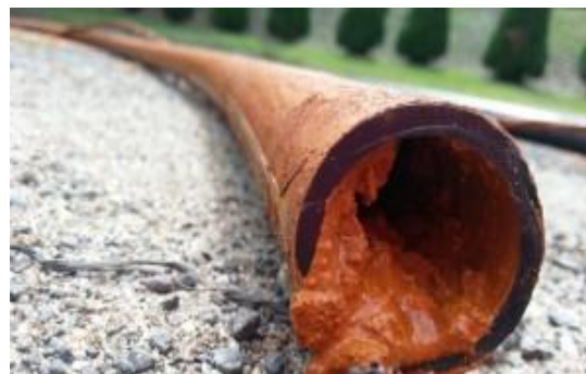
FIGURE 1 PIPE AFFECTED BY IRON BACTERIA
